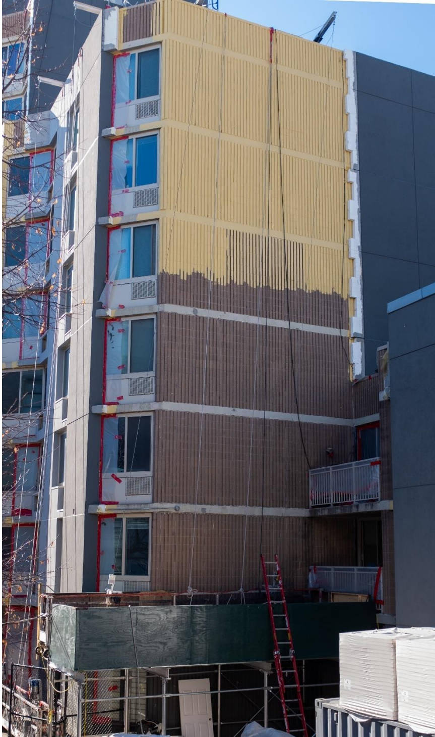
Figure 6: Metro North Riverview Apartments with in progress insulation installation. Original exterior is visible at bottom. Yellow coating (at top of wall) is applied to exterior before new cladding is added (large panels at right). (Author's photo)
