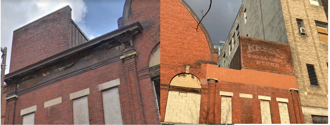
Figure 13. Left: Shows the original sheet metal cornice of the building. Corrosion caused discoloration to the surrounded bricks. Right: Shows cementitious coating on where the cornice was originally placed. Photographs by the author
