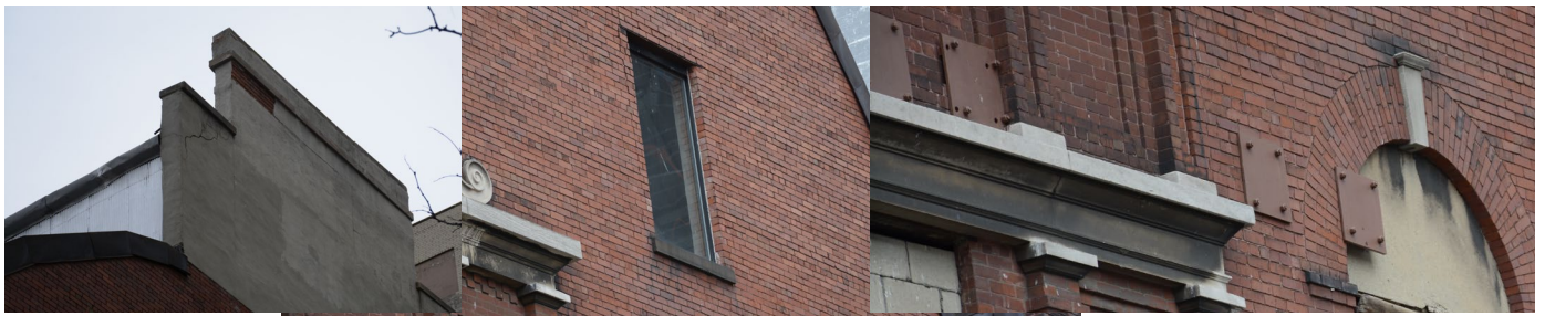
Figure 12. Left: Crack on the top part of the building with lost of coating. Middle: Minor crack around the window. Right: Anchors and Discoloration. Photograph by the author
