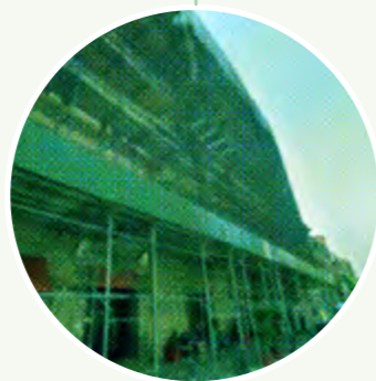
160 BLEECKER ST. As a scaffold erected for Local Law 11, it is 436 feet long and covers 24.18% of the sidewalk within the census block.
