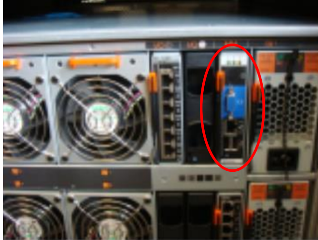
(BACK VIEW of IBM BLADE)
