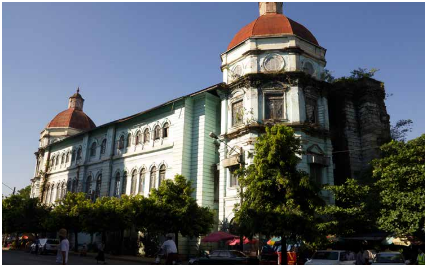
FIGURE 4. The Yangon Division Court building, circa 1900, was bombed during World War II and the damage is still evident.
