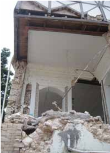
FIGURE 102 The horizontal metal ties within the masonry bearing wall probably kept this corner from collapsing entirely.
