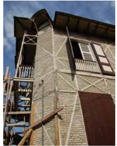
FIGURE 42 The house at 32 LaMartiniere. The braced timber frame and brick infill is a large component of the architectural vocabulary.
