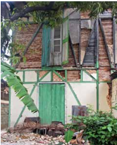
FIGURE 86 Much of the colombage stonework fell out of the walls of the second story during the earthquake.
