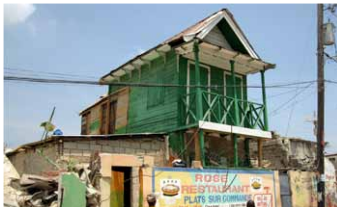
FIGURE 76 This two-story colombage house survived amid the collapse of numerous concrete buildings. The owners do not want to tear it down. However, it needs temporary stabilization and long-term repairs.
