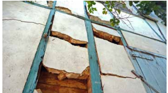
FIGURE 39 Colombage at 5 Rue Jose Marti with limestone and earth mortar infill, with lime plaster finish. Interior planking can be seen.
