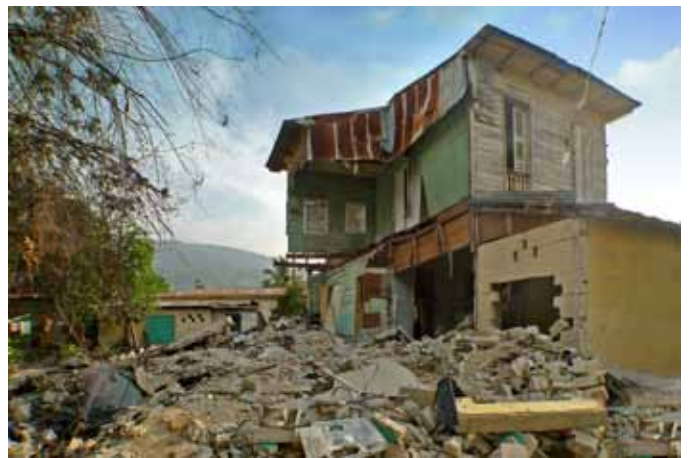
FIGURE 111 The wooden portion of this building remained standing, while the two-story concrete addition pancaked completely.
