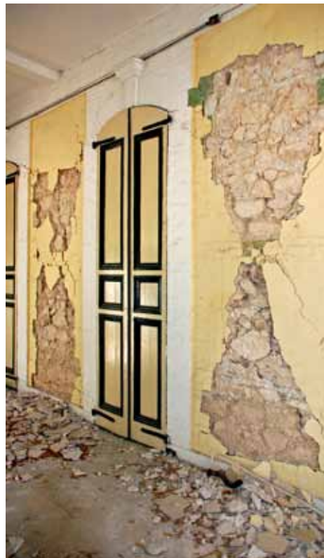
FIGURE 115 The characteristic X-cracks seen on masonry wall infills of concrete frames are also present at Le Manoir. These are due to the reinforced concrete second floor slab (above the damaged wall in this picture).
