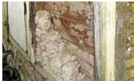
FIGURE 87 Close-up view of the failed colombage stonework. This infill, if laid up in clay, crumbles away and does not compromise the integrity of the wood braced frame.
