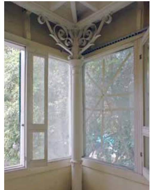
FIGURE 27 An example of the ornate metalwork in the second-floor balconies of La Manoir . This metalwork is obscured by wooden exterior walls.
