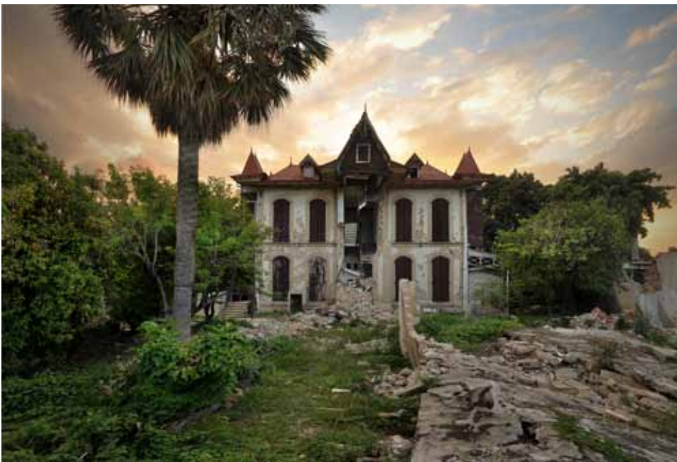
FIGURE 29 The east front of the Villa Castel Fleuri on Avenue Christophe, a grand brick and rubble stone masonry house. This house was occupied by the President of Haiti for a short period in its history. It has suffered extensive damage in the earthquake mainly to the projecting stair tower on the east side, and porches on the west. The plates that hold the iron ties that penetrate the building are visible on the façade.
