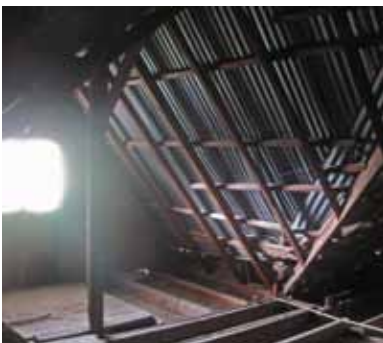
FIGURE 58 The wood structure of this attic would only incorporate a corrugated metal roof, indicating that these roof materials were original.
