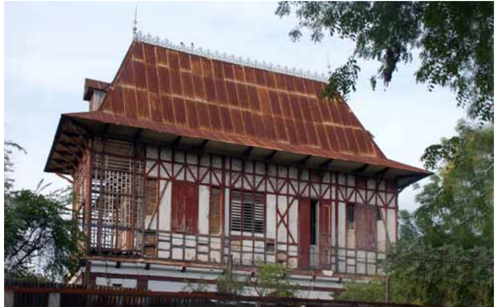
FIGURE 55 Corrugated ferrous metal roofs are quite common on the Gingerbread houses. This house has a metal crest at the ridge as well.
