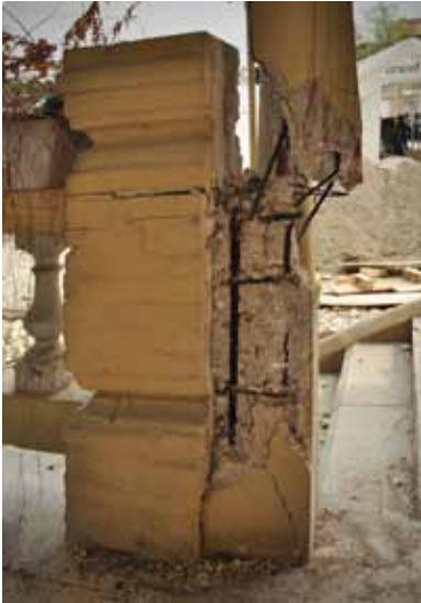
FIGURE 114 The Bazin House on Rue du Travail Deuxième. An upstairs bathroom of reinforced concrete and block construction clad with wood visible in the middle of the left photo almost caused the collapse of the entire house because it was standing on thin legs of heavily deteriorated concrete with rusted rebar. It was heavy, causing the whole house to sway, almost collapsing the bathroom wing, which may then have carried part of the house down with it.
