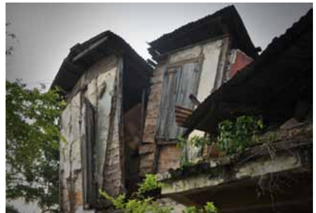
FIGURE 63 Heavily rotted and termite-eaten house on Avenue Lemartiniere, which partially collapsed during the earthquake.
