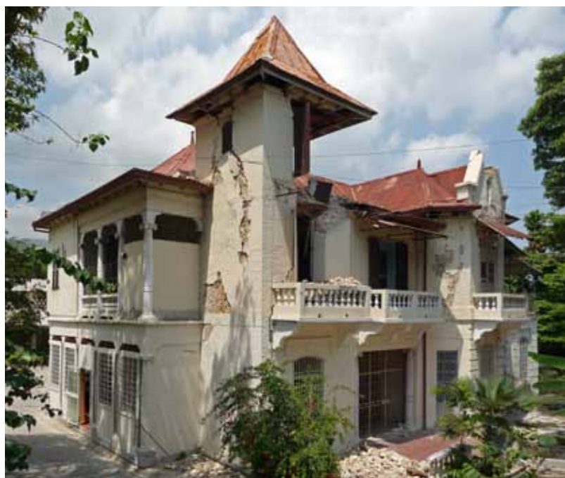
FIGURE 3 The Catholic seminary at 110 Rue Fleur Du Cheine. This masonry bearing-wall structure exhibits partial collapse of corner tower.
