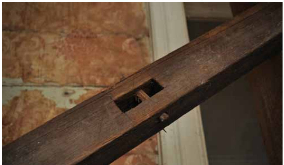
FIGURE 32 top The interior of a room constructed on what had been the porch of the Patrice Pamphile House at 4 Rue Casseus, shown in Figure 2. This interior shows the characteristics of the typical timber frame construction in Haiti, which lies somewhere halfway between the heavy timber framing with mortise and tenon jointing common in Medieval and Renaissance French construction, and the sawn light timber “balloon frame” of nineteenth-century American construction. bottom The example of the mortise and peg is from the Bazin House at 8 Rue du Travail Deuxième.
