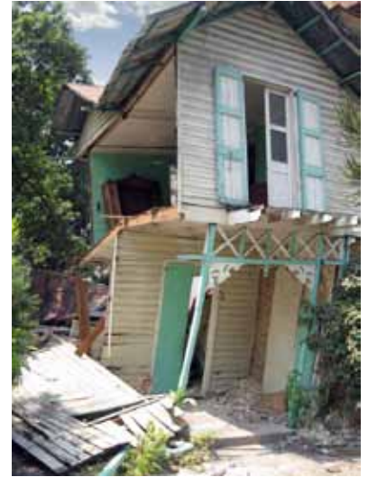
FIGURE 85 Despite severe damage, this colombage building did not fully collapse. Note that the wall that fell away is the one on the side parallel to the joists, thus not having substantial tie to the floor.
