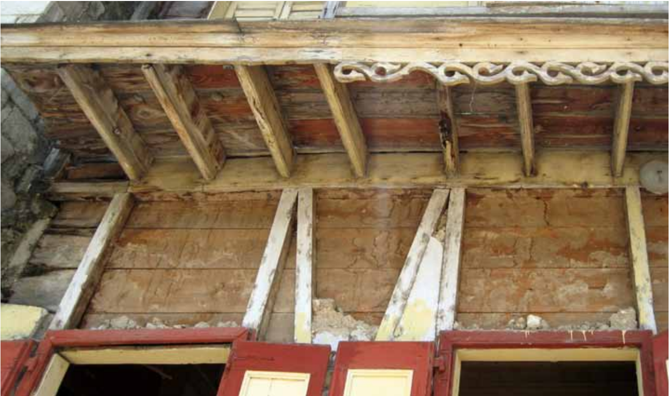
FIGURE 66 Some houses have cantilever balconies. These are vulnerable to decay at the critical location where the beams enter the wall.
