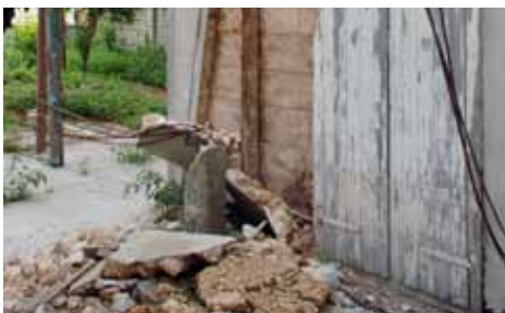
FIGURE 88 Stone infill that had been relaid with cement mortars would fall out of the wood frame voids in huge pieces during the earthquake causing damage also causing a safety hazard.
