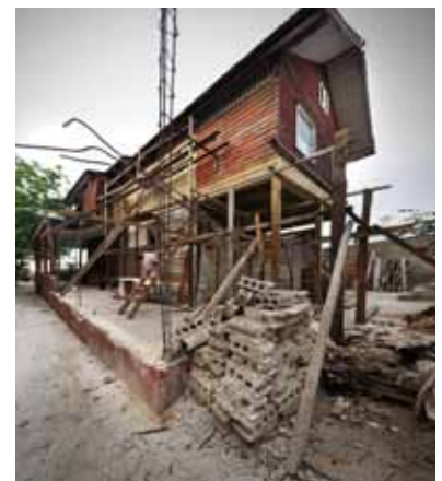
FIGURE 134 The modern reinforced-concrete frame with concrete-block back additions to the house at 24 Avenue Lamartiniere. The owner, architect Gilbert Mangenes, is now doing all of the repairs with timber framing and cladding, which will be much more compatible with the flexible timber frame of the original house, and less likely to collapse in a future earthquake.
