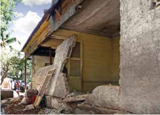
FIGURE 72 A replacement side wall of concrete block at 19 Lamar-tiniere suffered partial collapse.
