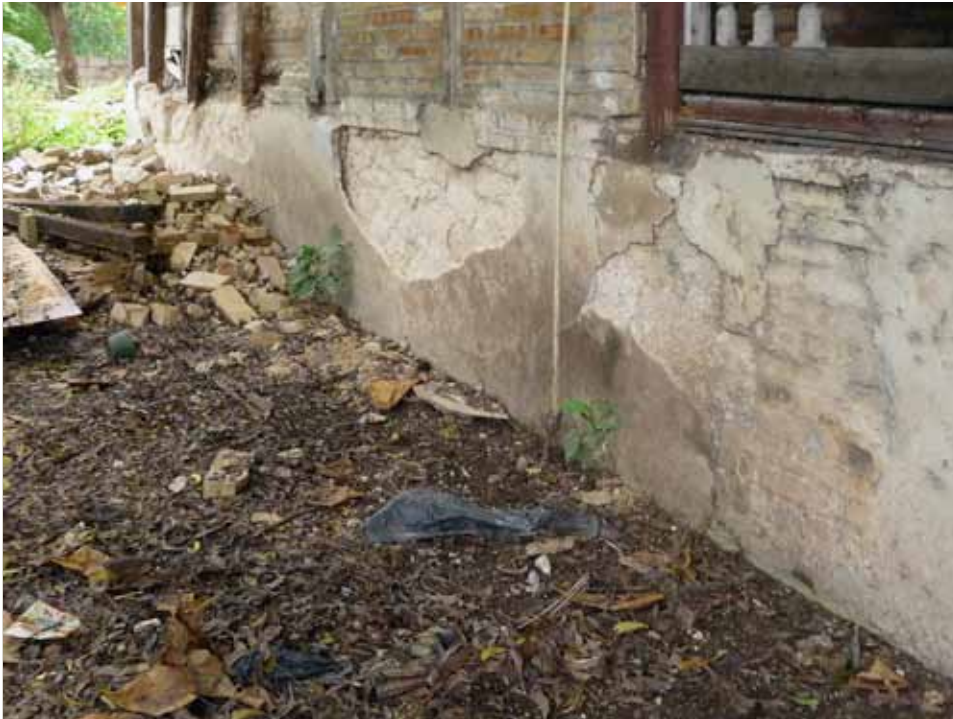
FIGURE 50 Spalling of the exterior finish plaster of the house at 84 Lamartiniere reveals two contiguous sections of foundation stem wall. One of irregular limestone left , and one of brick right .
