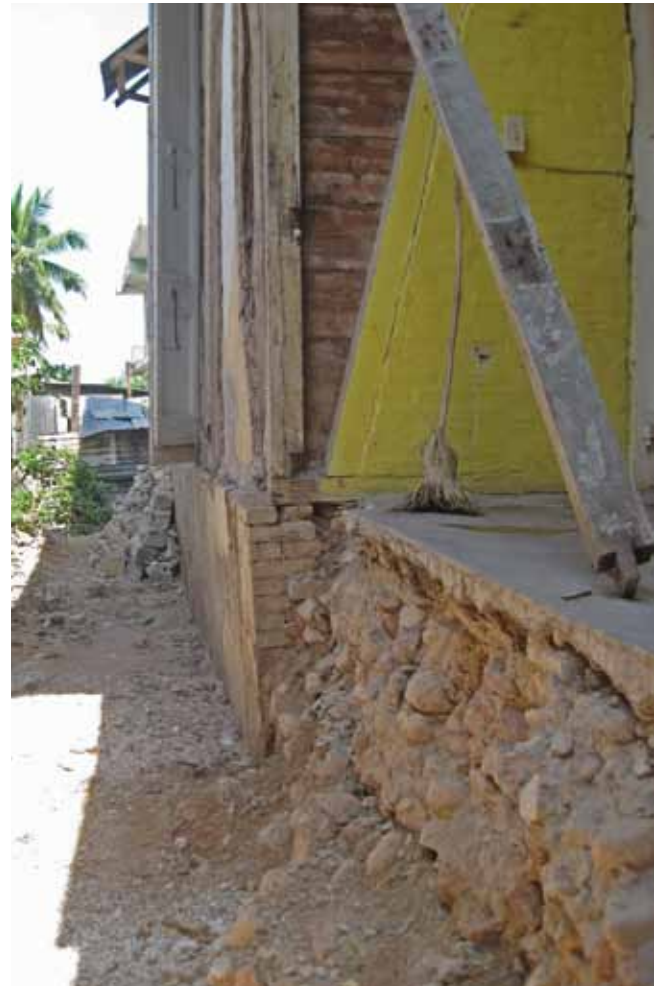
FIGURE 71 A portion of the foundation wall has collapsed at the house at 2 Avenue N, revealing that the crawl space below the first floor had been filled with rubble and the wood floor had been replaced with a slab on grade. Lateral loads on the wall from the fill caused it to collapse. The foundation wall remaining has rotated outward.
