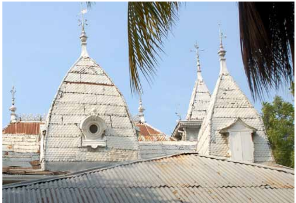
FIGURE 56 The roofs of the turrets of La Manoir utilize decorative pressed metal roof shingles.
