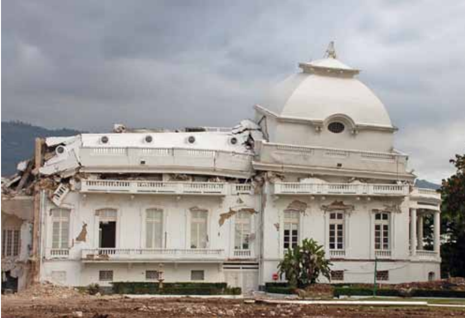
FIGURE 28 The Palais Nationale , constructed in 1918, is an example of early reinforced concrete use in Haiti. These buildings typically collapsed.
