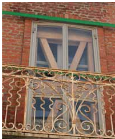
FIGURE 138 Examples of shoring constructed after the two recent earthquakes in Italy demonstrate different solutions to the important problem of stabilizing heritage structures to avoid emergency demolition for public safety. The two photos on this page show an unreinforced masonry building damaged in the 2002 Molise earthquake shored entirely with polyester straps, thus eliminating the need to block the street with diagonal braces. Shoring has been installed in the window openings—an important part of any system as it gives the damaged masonry wall structural continuity across openings.
