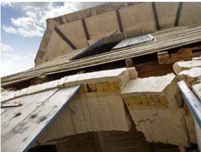
FIGURE 105 Severely damaged arch, and displaced wood framing above. Absence of tie rods, combined with decay of the timber sill plates made the building more vulnerable.
