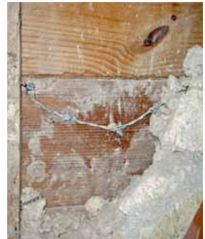
FIGURE 125 Barbed wire is frequently seen in the wall cavities as a restraint for the rubble fill. This is a good practice and should be continued.
