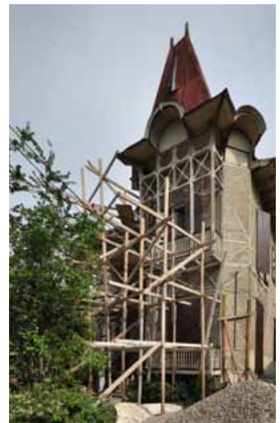
FIGURE 120 Scaffolding and shoring at 32 Lamartiniere, and shoring on the interior of 22 Rue Pacot.
