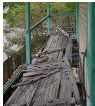
FIGURE 78 Second-floor porch structure made unsafe by termite damage.
