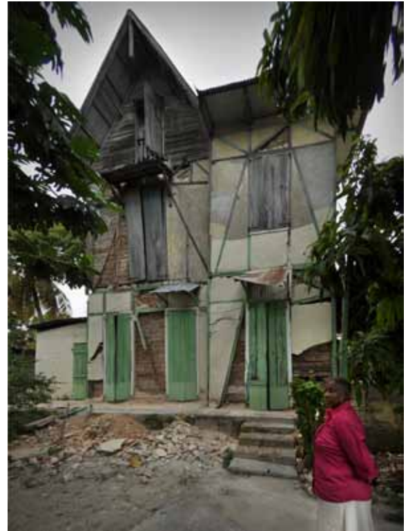
FIGURE 83: Marie Céleste Florence Jacob, seen here, continues to live in this century-old wood frame house at 14 Rue Marcelin. This house was extensively consumed by termites prior to the earthquake which damaged it further. Even in this badly compromised state, this structure remained standing after the earthquake only a few short blocks away from the National Palace and many other concrete frame structures which collapsed.
