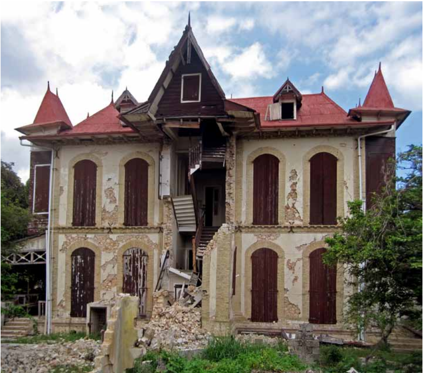
FIGURE 47 View of the back elevation of Castel Fleuri. The use of brick masonry surrounding the windows, at the corners, and at floor lines in tandem with the stucco over the stone masonry elsewhere forms a pleasing composition.
