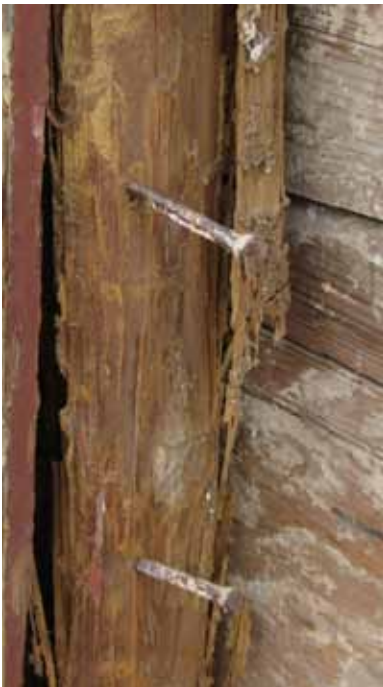
FIGURE 84 Despite extensive termite damage, the remainder of this post is hard and dense, still holding the nail firmly.
