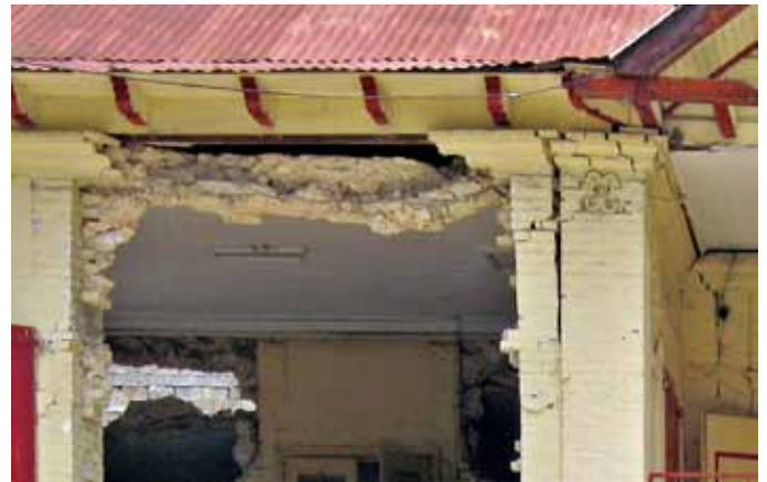
FIGURE 104 Total collapse was avoided in this heavily damaged masonry building due to embedded iron rods at the top of the walls, with exposed end plates.
