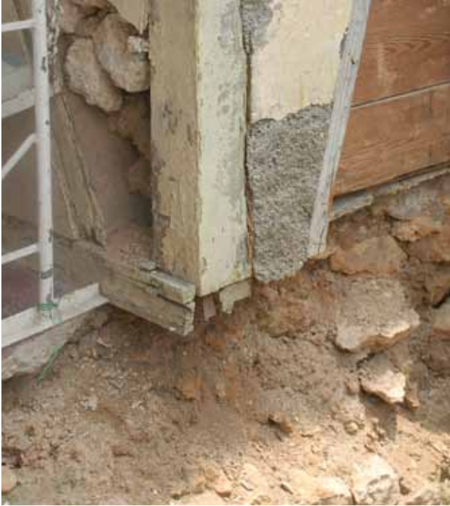
FIGURE 79 The wood sill that was previously termite damage crushed during the earthquake causing the entire structure to settle on its foundation. The result is that many of the doors to the exterior cannot be opened or closed.
