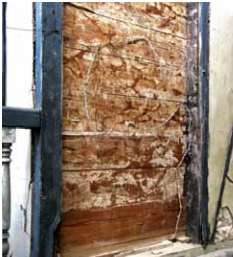
FIGURE 40 In this colombage construction the stone infill has collapsed due to the earthquake revealing the barbed wire reinforcement. This is an example of a non construction material being adapted for construction due to its apparent availability. The barbed wire was galvanized and is still in good condition.
