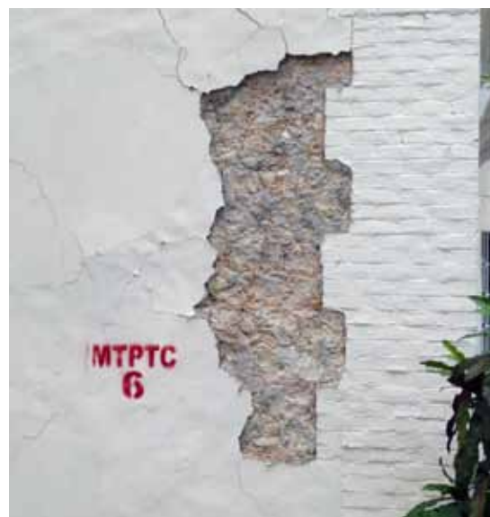
FIGURE 4 The red painted designation “MTPTC 6” indicates that inspection deemed the tower unsafe for occupancy by the Ministère du Travail Public et Télé Communications.
