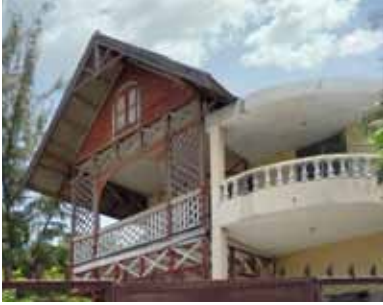
FIGURE 48 Concrete additions are often awkward or compromise the Gingerbread buildings architecturally, like this one at 51 Avenue Christophe.
