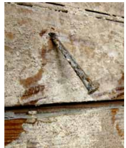
FIGURE 81 Cut nails of iron or steel are common in the Gingerbread houses. Many of the original cut nails show surprisingly little corrosion.
