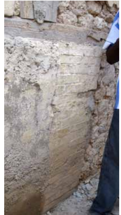
FIGURE 51 The original brick masonry foundation pier can be seen and is infilled on either side with stuccoed stonework.
