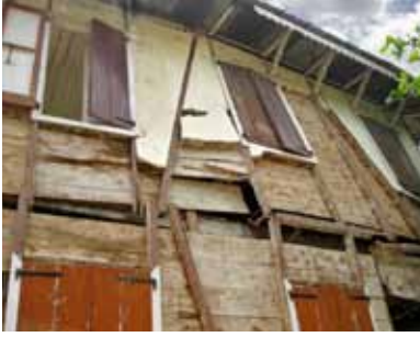
FIGURE 123 Typical vulnerability: the wall pulls away on the side parallel to the floor framing due to lack of connectivity between the floor and the wall. This is easily improved in most houses.
