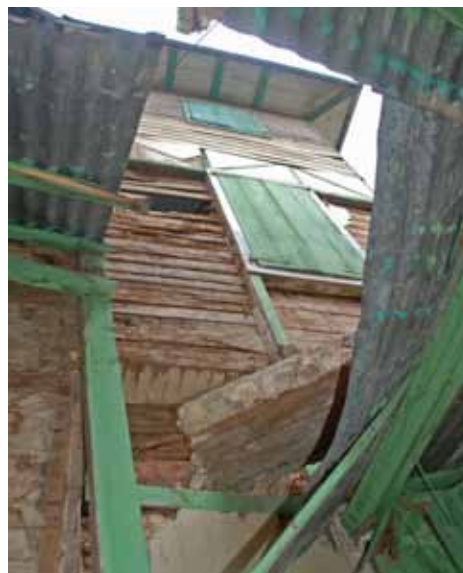
FIGURE 89 Brick infill that had been relaid with cement mortar fell out in huge pieces during the earthquake, causing damage to construction below.
