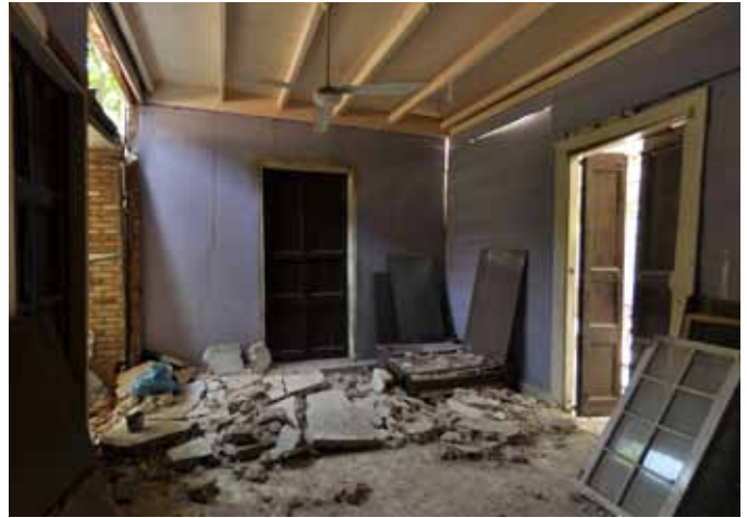
FIGURE 73 These are examples of colomage where the rubble infill has been replaced with concrete. This has accelerated the rotting of the timber framing, which then broke during the earthquake causing the collapse of the heavy concrete infill.
