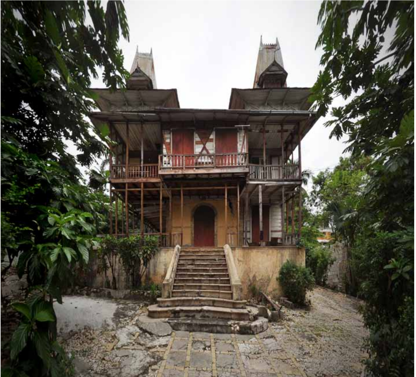
FIGURE 1 cover: The west front of the Villa Castel Fleuri on Avenue Christophe, a grand brick and rubble stone masonry house. This house was occupied by the President of Haiti for a short period in its history. It has suffered extensive damage in the earthquake mainly to the projecting stair tower on the east side, and porches on the west. The plates that hold the iron ties that penetrate the building are visible on the façade.
