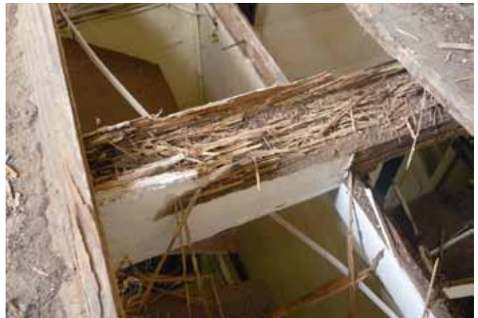
FIGURE 68 Termite damage in second story floor joists.
