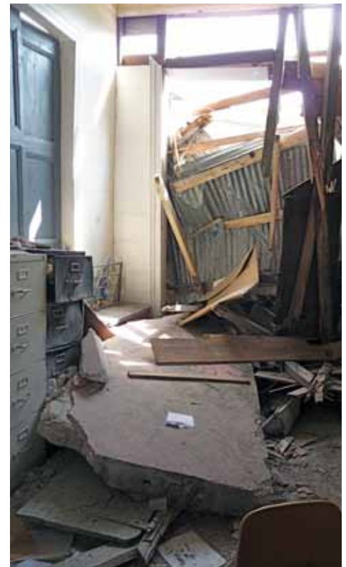
FIGURE 116 The most damage this building suffered was from a concrete slab ejected through its back door from the collapsed concrete building behind.
