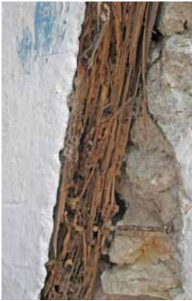
FIGURE 62 Termites thrive in Port-au-Prince, and many of the wooden structures are severely damaged due to termite attack.
