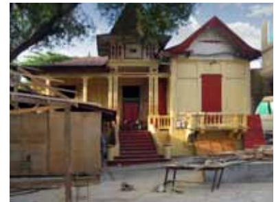
FIGURE 30 Concrete frame/confined masonry Gingerbread. This is the only variant of this type seen. It was undamaged.
