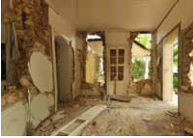
FIGURE 94 Ground floor interior of the Albert Dufort House on Rue du Travail Deuxième showing complete disruption of the rubble panels in its construction. The interior wall on the left, which did not have brick piers walls because of the lack of window and door openings, collapsed completely.
