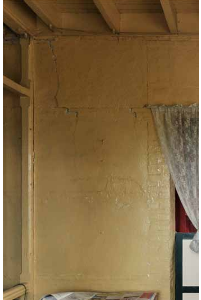
FIGURE 128 Interior and exterior examples of low levels of damage to rubble stone panels in masonry walls.
