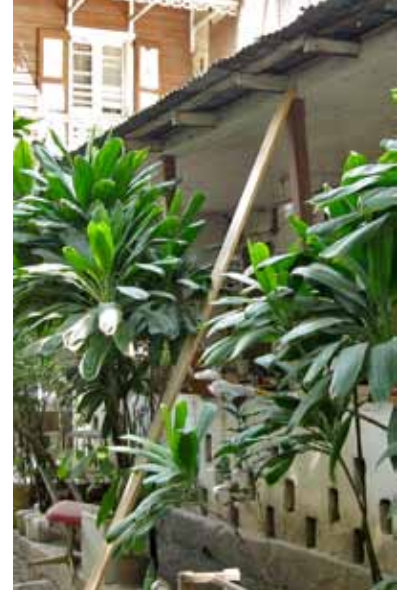
FIGURE 119 Temporary measures are important: this lateral brace is a good idea, but it is too slender and there is only one.
