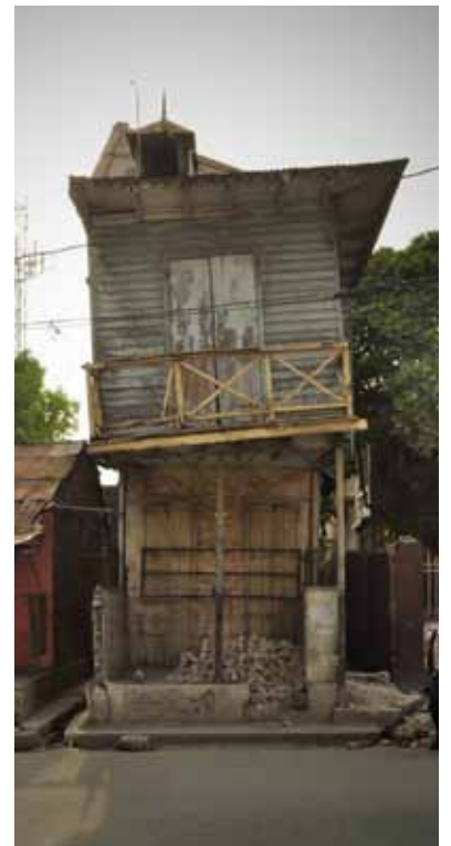
FIGURE 90 A wood clad and colombage structure of the most basic type on Rue Geffard near the National Palace. This structure appears to have been designed to be expanded to double its width, but never was. As a result, it was subject to the earthquake with a width at the base of less than 12 feet (3.6 meters). Also, at the time of the earthquake, it was in extremely poor repair. In spite of all of this, the earthquake did not cause it to collapse.
