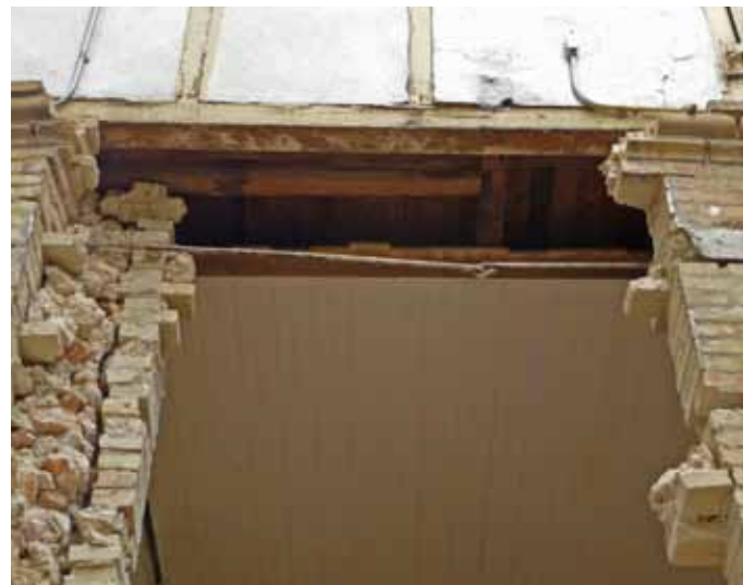
FIGURE 106 Linked iron tension rods exposed after the limestone infill panel was discharged. The rod may have prevented complete wall collapse.
