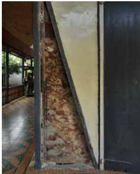
FIGURE 41 House at 15 Rue M showing plastered rubble stone infilling. On the left, one panel fell out in the earthquake, revealing that it was reinforced with barbed wire inserted into the bay in a zigzag layout.
