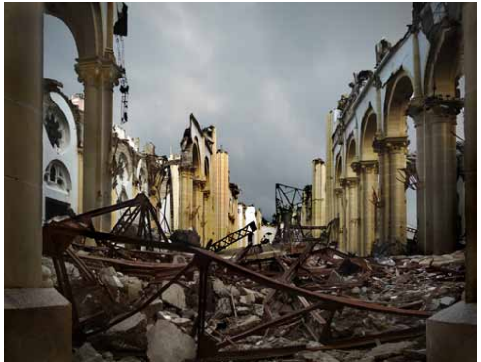
FIGURE 131: interior of the Cathédrale Notre Dame de L'Assomption after the 2010 earthquake collapsed much of its walls, almost all of its roof, and the tops of both towers. The building was constructed between 1884 and 1914, with walls of reinforced concrete with infill masonry construction. Much of the reinforcing had become heavily corroded by the time of the earthquake.
