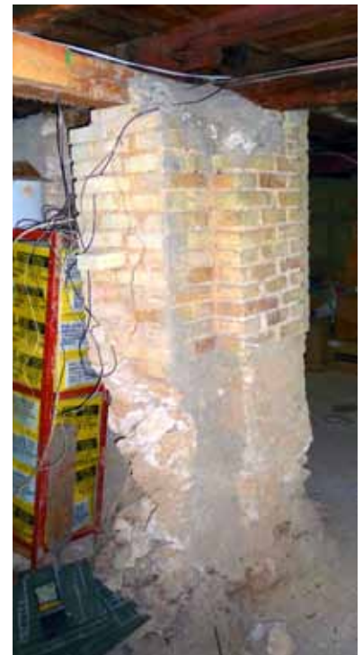
FIGURE 52 An excavated crawl space in the house at 84 Lamartiniere shows an original above-grade brick pier, and its uncovered, original limestone and earth mortar footing.
