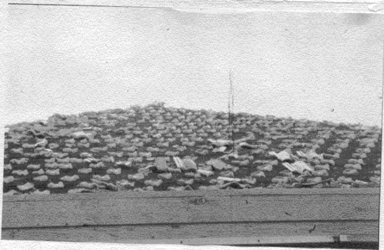
Photo 8 - Loss of precast-concrete, barrel tiles (Andrew, Florida)
