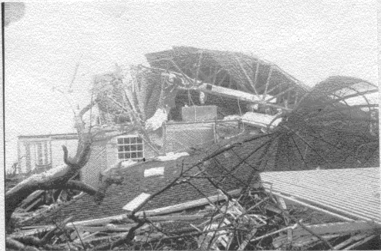
Photo 4 - Destruction of expensive, timber-framed residence (Andrew, Cat Cay, Bahamas)
