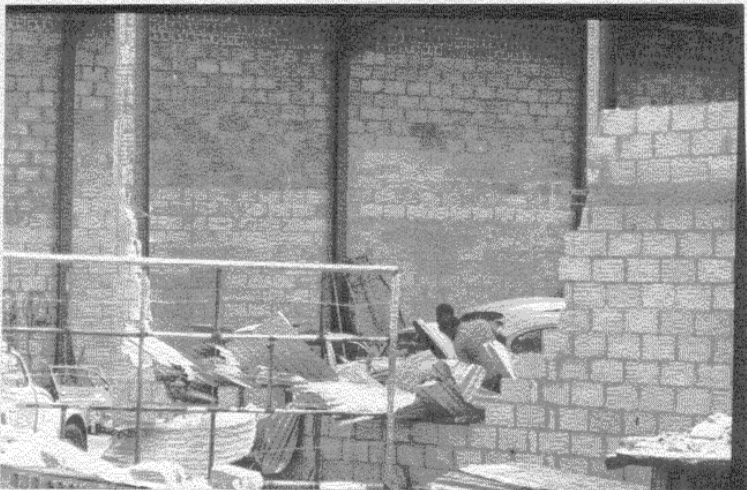
Photo 11 - Breaching of unreinforced blockwall (David)
