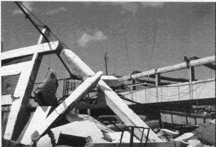
Photo 5 - Destruction of reinforced-concrete frames (David)
